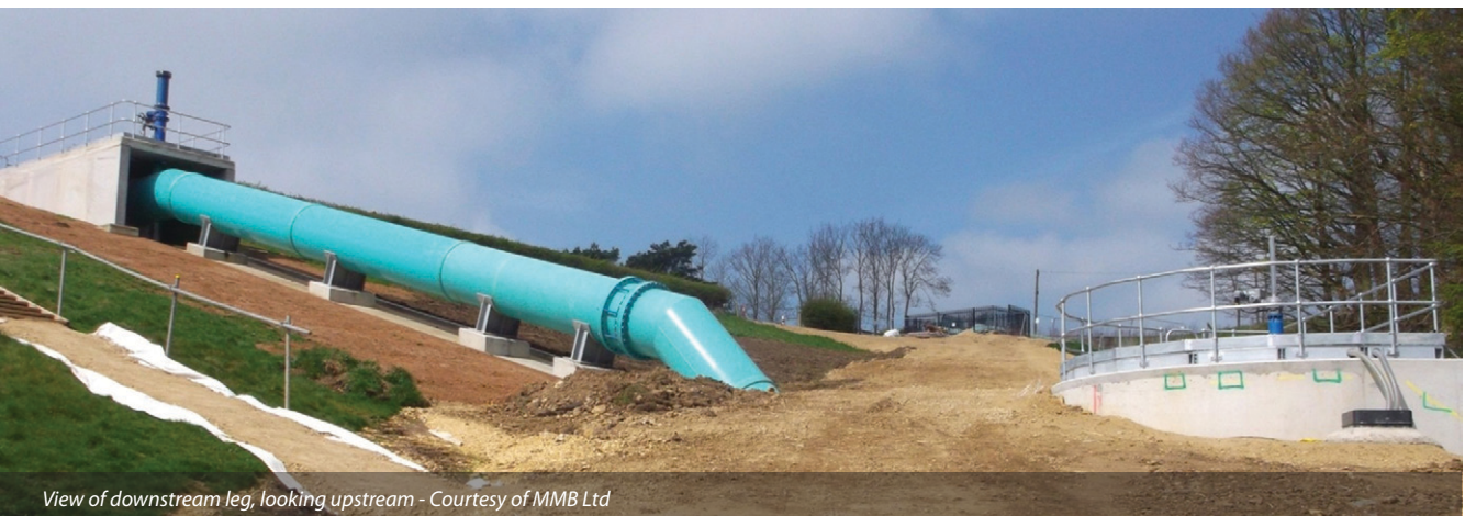
Discharge chamber - Courtesy of MMB Ltd
