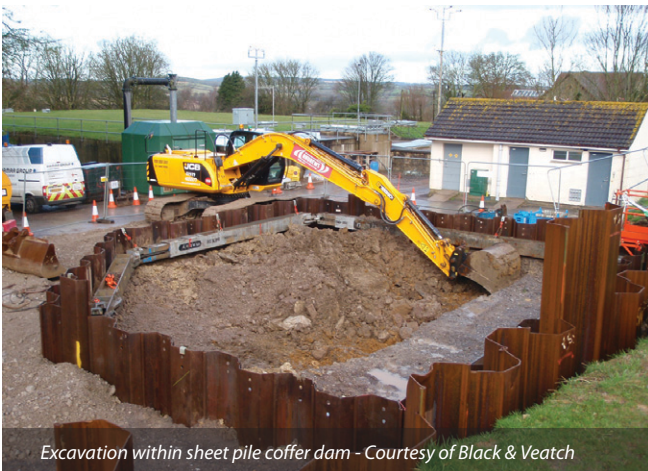
Site constraints: construction of PS in close proximity to existing plant Courtesy of Black & Veatch
