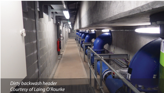
Design Engineered model. Positioning valve actuators along length of the walkway to maximise access - Courtesy of Laing O'Rourke
