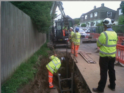
Checking distance of overhead cables Courtesy of HsO
