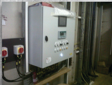
New control panel Courtesy of HsO
