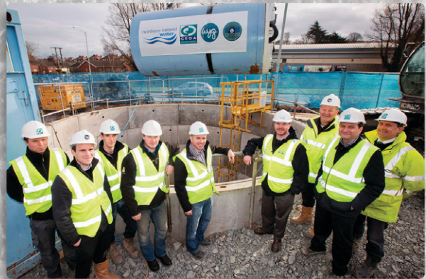
Members of the project delivery team with tunnel boring machine in the background - Courtesy of NI Water
