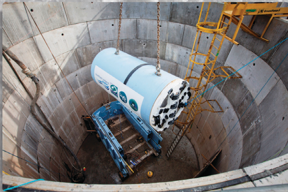
Tunnel boring machine being lowered into position for first tunnel drive Courtesy of NI Water
