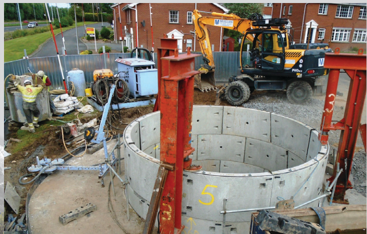
Construction of segmental shaft manhole at Strathearn Court, Holywood - Courtesy of NI Water
