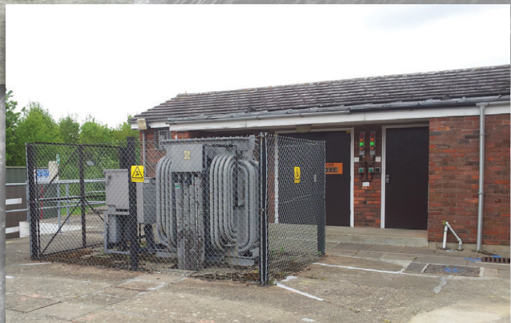
Existing ASR1 LV substation and MCC at ASR1 - Courtesy of Mott MacDonald
