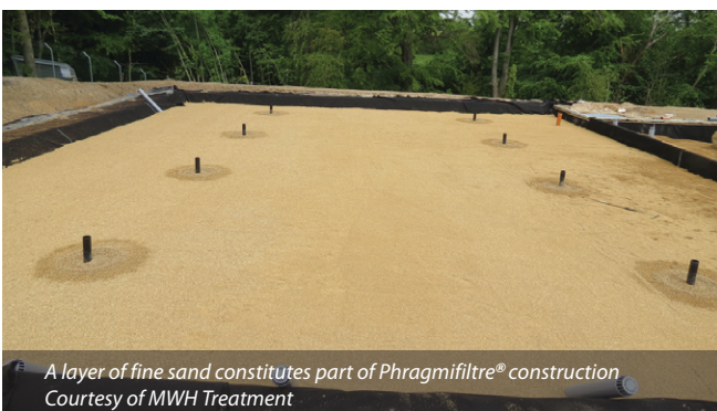
ARM employees rake the sand on to the base of the reed primary beds 1 & 2 - Courtesy of MWH Treatment
