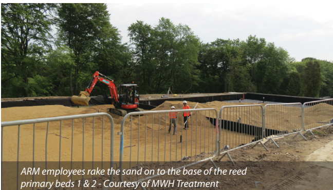
Excavators are used to lay the sand on top of the gravel Courtesy of MWH Treatment
