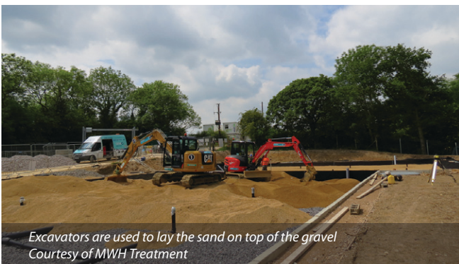
The base completed secondary reed beds can be seen in the distance with the 1960s conventional treatment works at the front - Courtesy MWH
