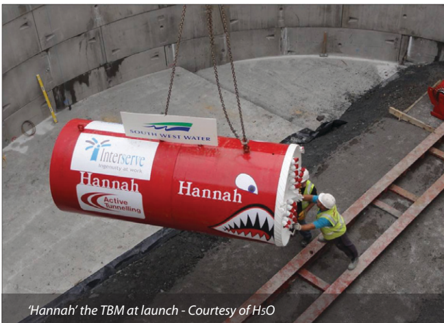
The 15m diameter storm tank whilst tunnel boring was under way. The TBM was launched from the tank – Courtesy of H5O
