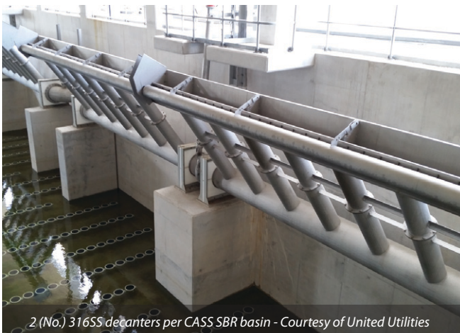
The Liverpool project was at the forefront of BIM technology Courtesy of United Utilities
