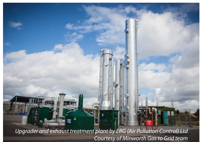
Removing the contaminants: showing all of the processes for trace element removal - Courtesy of Minworth Gas to Grid team
