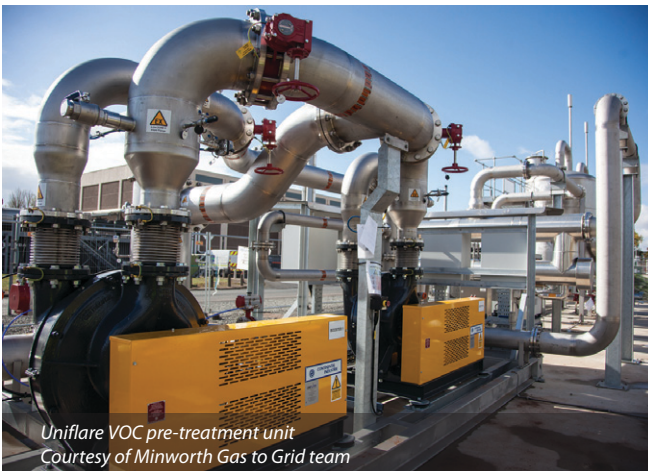
Final Polishing tanks (medium pressure activated carbon) to prevent pass through of chemicals into the grid - Courtesy Minworth Gas to Grid team
