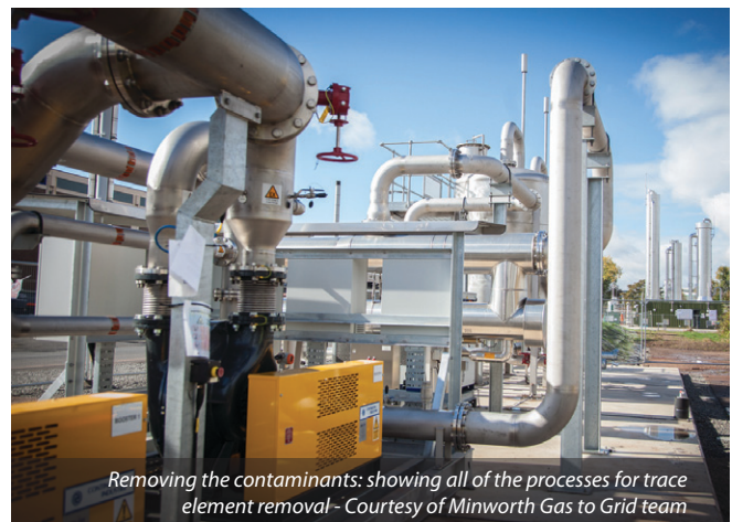
Internal plant room for Malmberg Upgrader: compression plant for the water scrubber - Courtesy of Minworth Gas to Grid team
