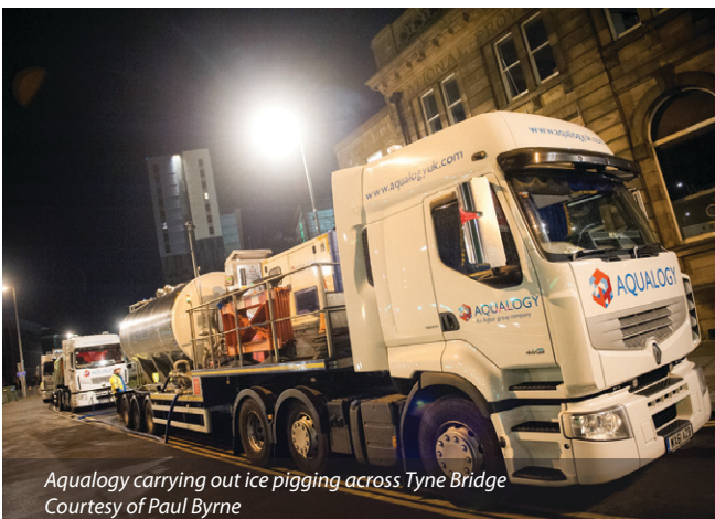
Fastflow cleaning head first pass entering 24' epoxy lined pipe, 03/2009 Courtesy of Northumbrian Water
