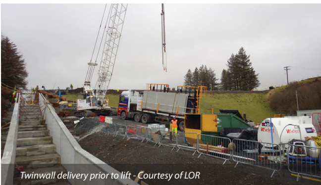
Step spillway bases, prior to pouring infill stitches and anchoring Courtesy of Laing O'Rourke
