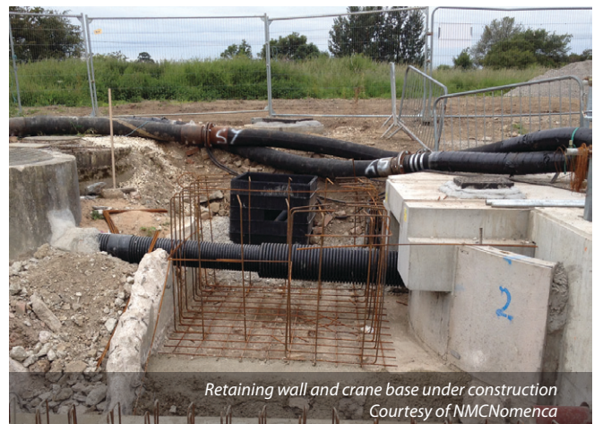
View across refurbished site showing new surge vessel and crane Courtesy of NMCNomenca
