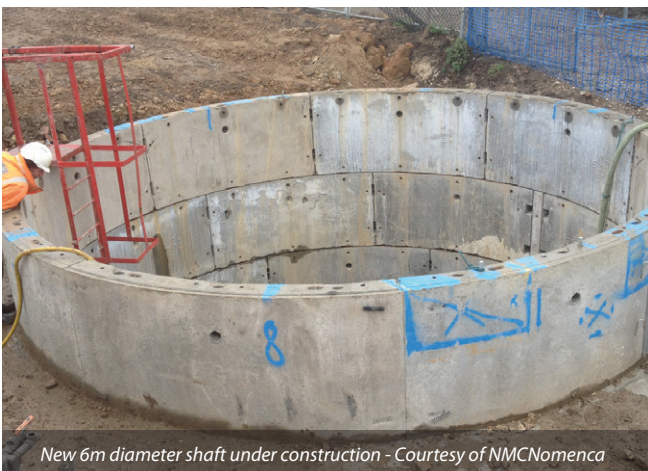
Breaking out of old storm overflow chamber in preparation for new shaft - Courtesy of NMCNomenca
