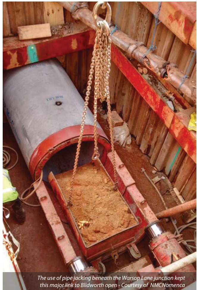
Extensive liaison with Nottinghamshire County Council highways aimed to minimise disruption to traffic - Courtesy of NMCNomenca
