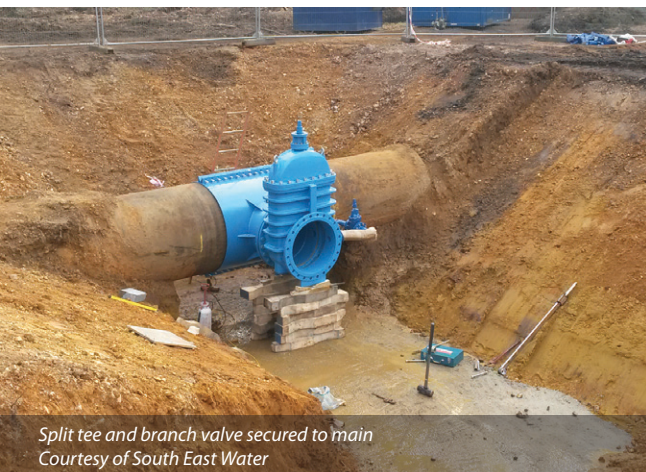
Cutting head post drilling with coupon still inside Courtesy of South East Water
