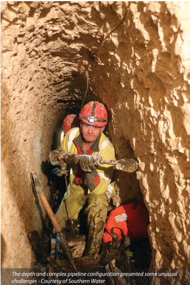
Underground engineering specialists were employed and bespoke systems were created - Courtesy of Southern Water
