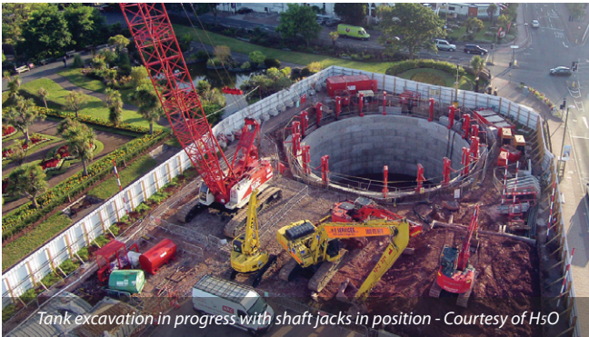
Third ring of total of 11 in position, 23T excavator excavating for next ring, long reach excavator removing spoil - Courtesy of H5O
