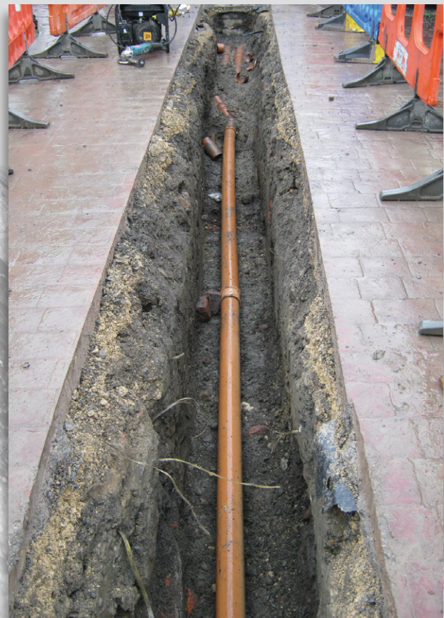
Existing pipework - Courtesy of Grontmij
