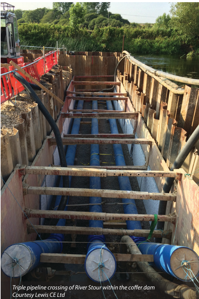
Lewis CE Ltd pipe laying gang progressing along the easement, the material laid out ahead of them - Courtesy of Wessex Water
