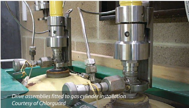
Gas detection sensors in the gas store - Courtesy of Chlorguard
