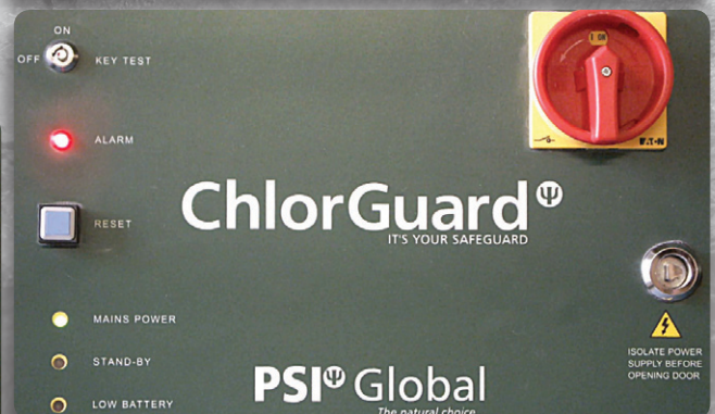
Chlorguard activation points - Courtesy of Chlorguard
