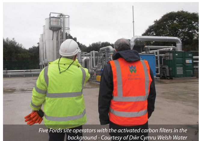
Activated carbon filters, and in the background, the screw compressor and membrane kiosk - Courtesy of Dŵr Cymru Welsh Water
