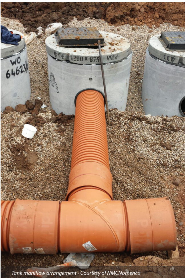
DN1200 concrete end entry manholes positioned in the trench Courtesy of NMCNomenca
