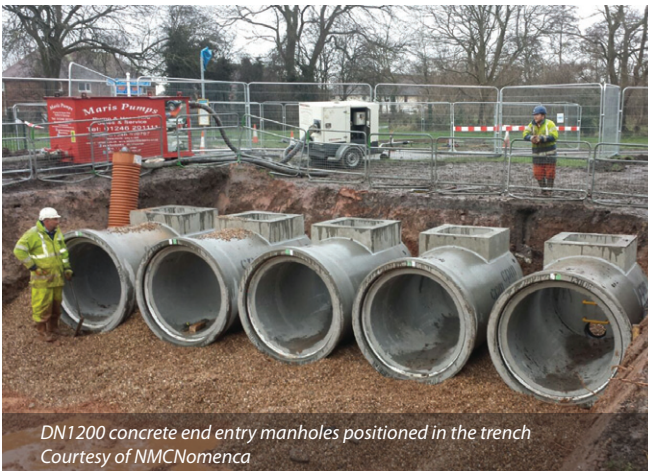
Battered excavation with concrete pipes partially backfilled with gravel Courtesy of NMCNomenca
