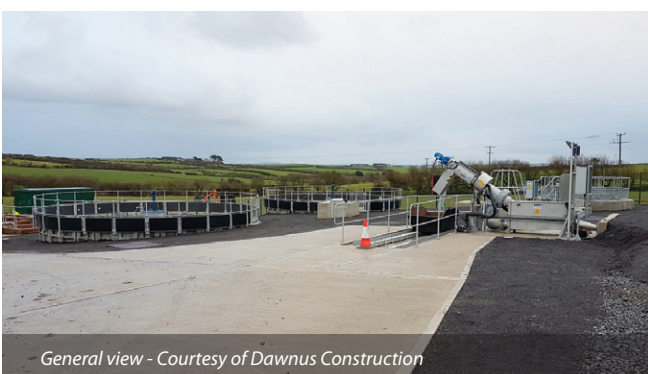
Filter bed with storm tank in the background Courtesy of Dawnus Construction
