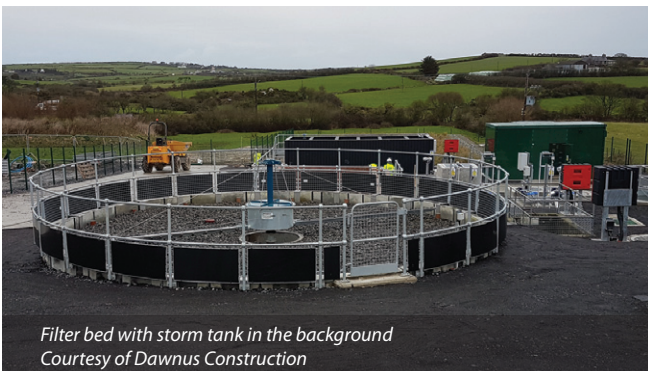
General view from primary tank over the site before stone dressing to surface - Courtesy of Dawnus Construction
