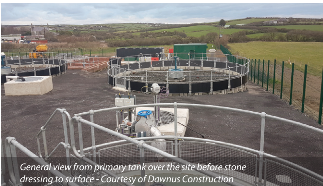
Humus tank and works return pumps looking toward MCC Courtesy of Dawnus Construction
