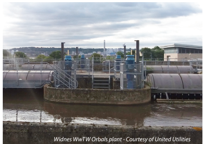
Bolton WwTW activated sludge plant - Courtesy of United Utilities
