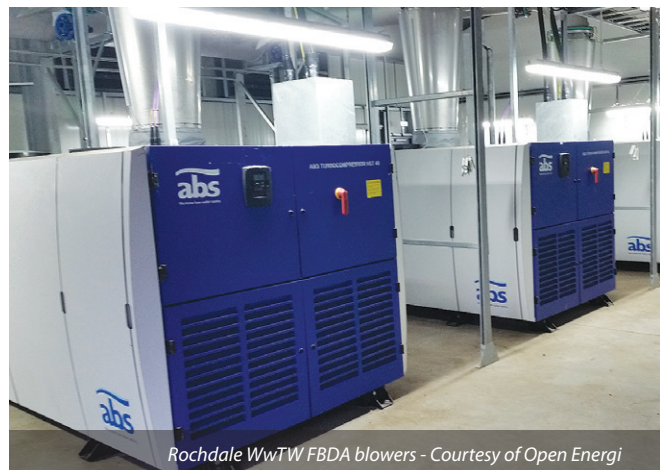
Rochdale WwTW FBDA plant - Courtesy of United Utilities
