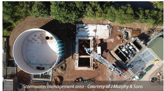
Inlet works - Courtesy of J Murphy & Sons
