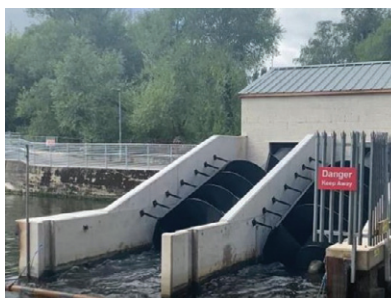
2 screw generators supplied, installed and commissioned for a hydropower generation scheme
