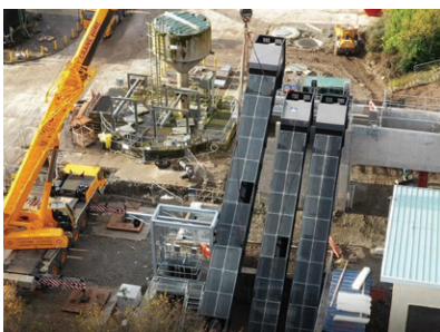
3 compact screw pumps supplied, installed and commissioned for a sewage treatment works
