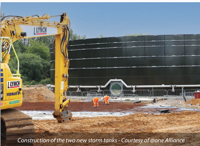
Terminal pumping station pipework to storm tanks Courtesy of @one Alliance
