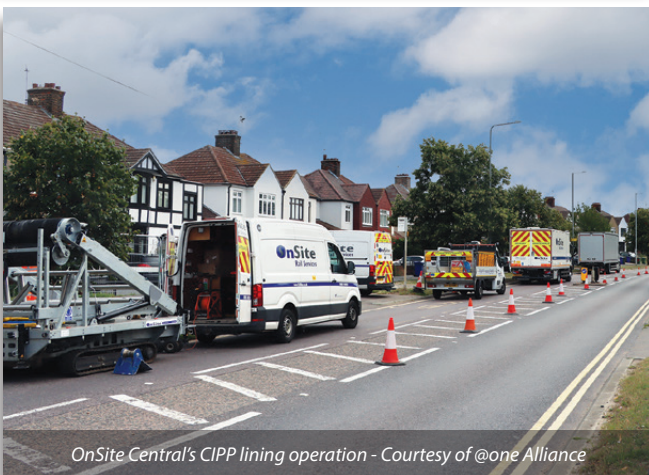
Overpumping pipework - Courtesy of @one Alliance
