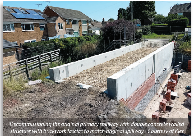
The original upper draw-off inlet has been discontinued by grouting up the inlet and full pipe running through the embankment - Courtesy of Kier
