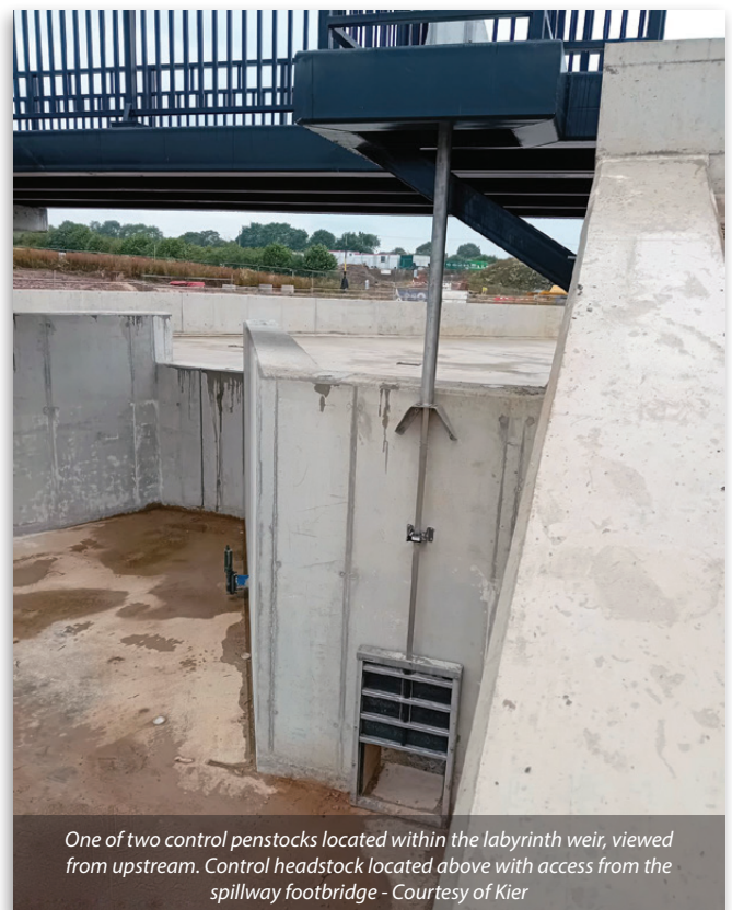
Access and water control for the reservoir team to operate the penstocks within the new labyrinth weir. Wheel is lockable to prevent unauthorised use - Courtesy of Kier
