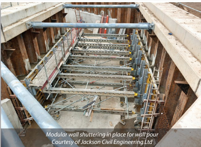
Excavated fish pass awaiting FRC works Courtesy of Jackson Civil Engineering Ltd
