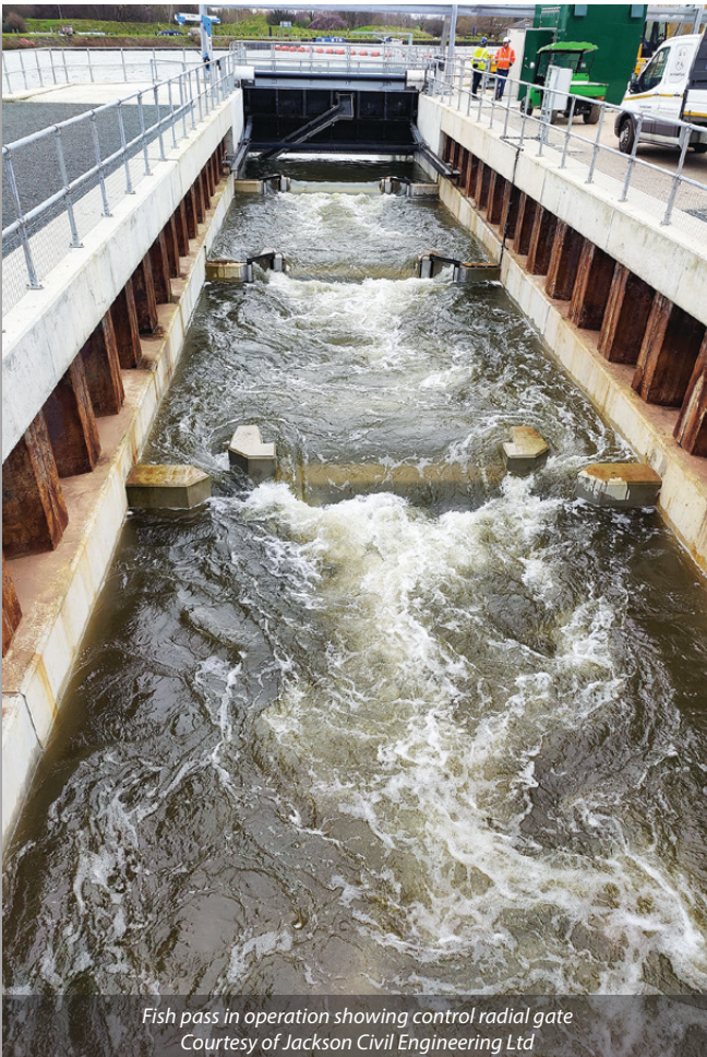
Completed fish pass looking towards the intake structure Courtesy of Jackson Civil Engineering Ltd
