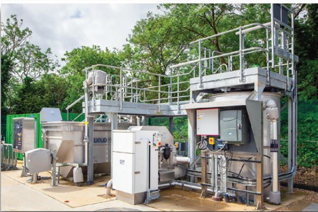
Tertiary solids removal plant - Courtesy of EPS Water
