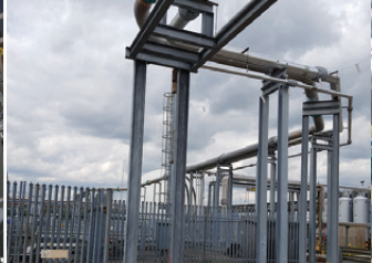
Pipe Bridges & Supports
