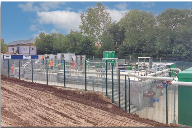
View of the main MBBR treatment block - Courtesy of EPS Water
