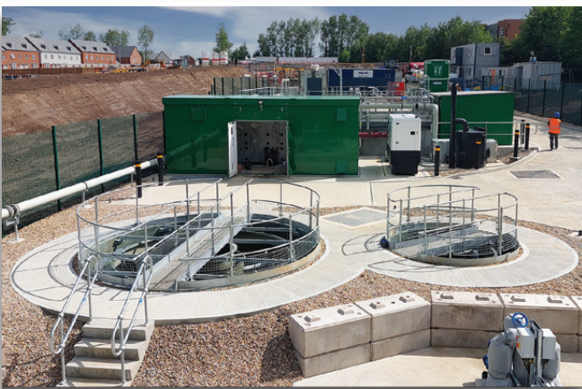
View of the clarifier, sludge thickener & MCC kiosk - Courtesy of EPS Water
