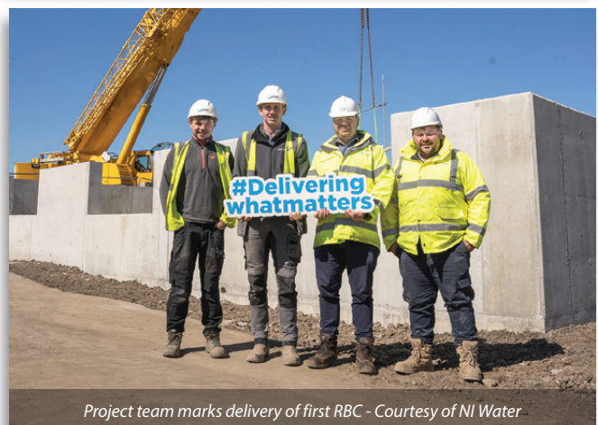
Construction of inlet works, sludge tank & storm tank - Courtesy of NI Water
