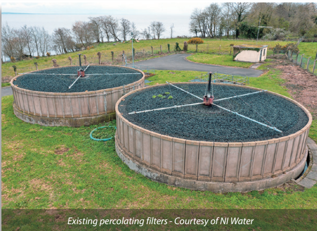
Existing site on western shores of Lough Neagh - Courtesy of NI Water
