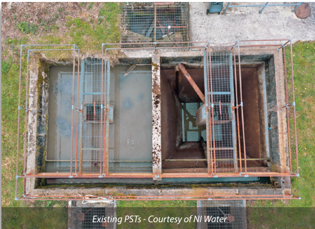
Existing percolating filters - Courtesy of NI Water
