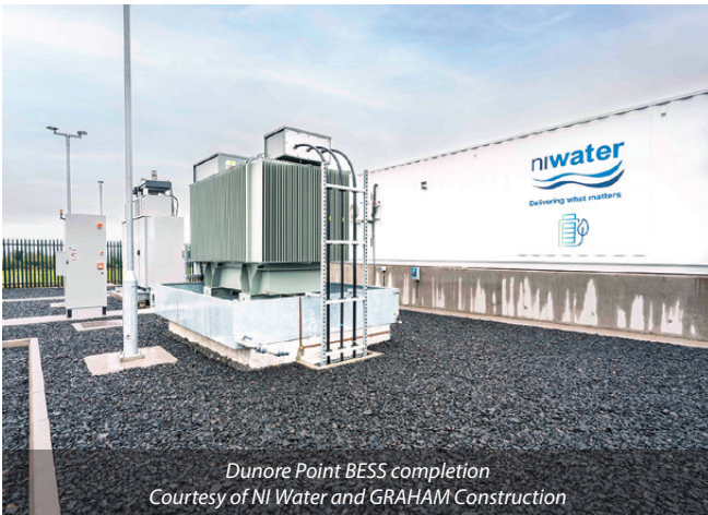
Dunore Point BESS completion Courtesy of NI Water and GRAHAM Construction
