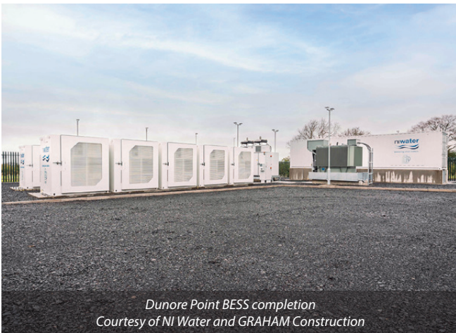
Inside of BESS cubicles and gridstack layout Courtesy of NI Water and GRAHAM Construction
