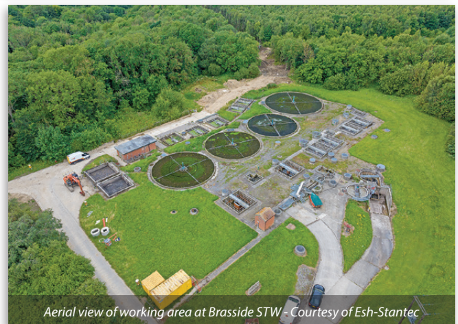
Construction of new valve chamber and associated pipework at Pity Me STW Courtesy of Esh-Stantec
