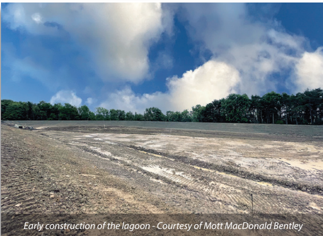
Field where the lagoon will be sited - Courtesy of Mott MacDonald Bentley
