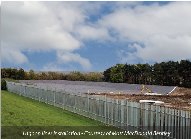
Security gate installed to allow access to lagoon area - Courtesy of MMB
