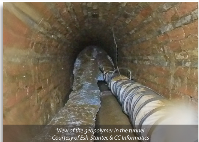
View of pipe inlet and partial headwall. Notice standing water on the invert of the tunnel - Courtesy of Northumbrian Water & Academy Geomatics
