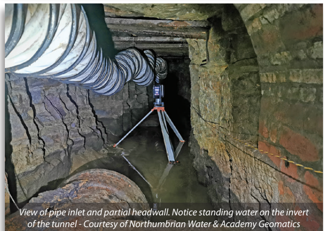
View in the unlined section of the tunnel (notice the beams across the soffit) Courtesy of Northumbrian Water & Academy Geomatics
