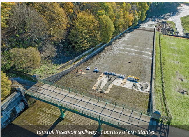
Overview of the siphon diversion route in preparation for the works Courtesy of Esh-Stantec
