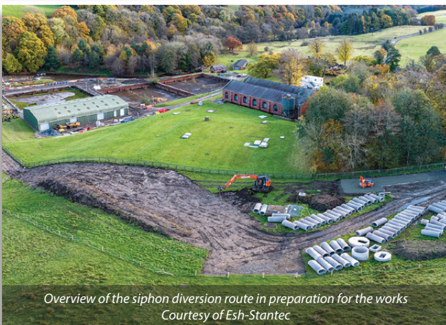
(left) Condition of the spillway blocks prior to the works & (right) new concrete slab with stainless steel protection to the joint - Courtesy of Esh-Stantec
