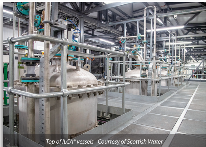
Raw water pumps and tank - Courtesy of Scottish Water
