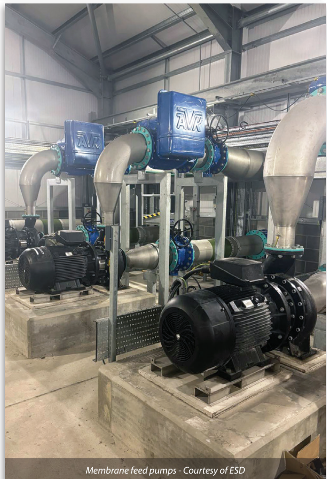
Expansion to membrane plant - Courtesy of ESD
