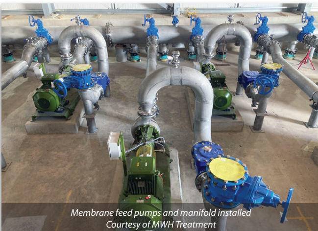
CeraMac C90 and backwash vessel Installation Courtesy of MWH Treatment
