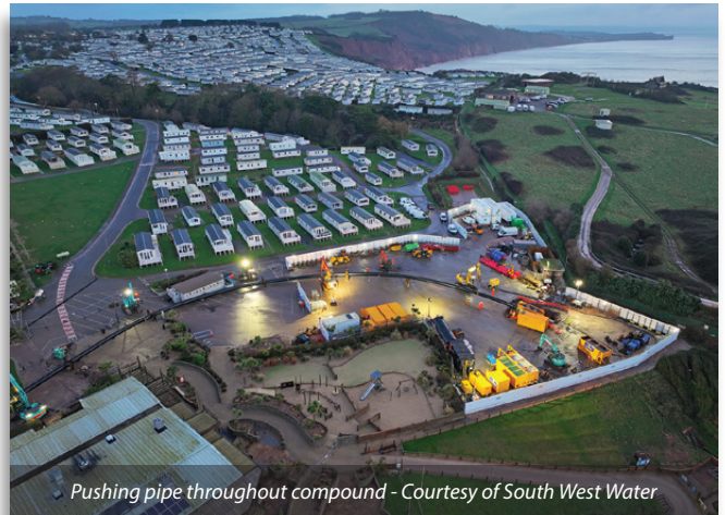
Pushing pipe lower car park and compound - Courtesy of South West Water
