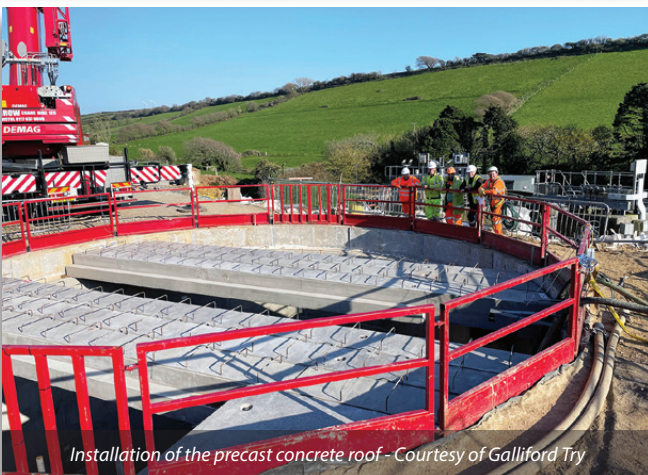
Inside the Galmpton stormwater storage tank - Courtesy of Galliford Try
