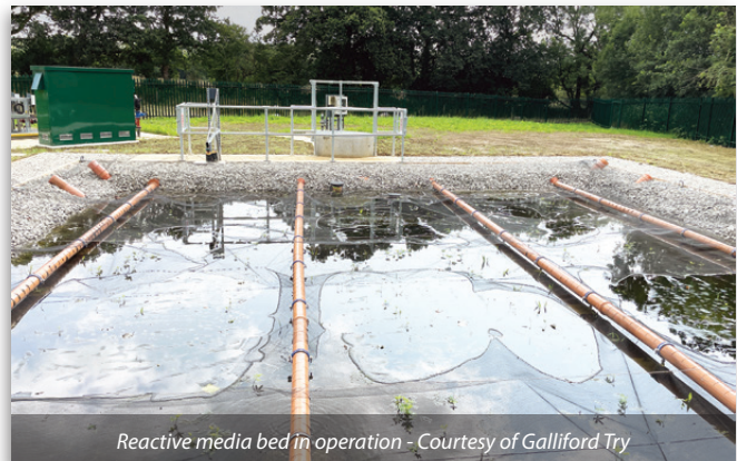
Phosphate removal process added to the works as a new tertiary treatment process - Courtesy of Galliford Try
