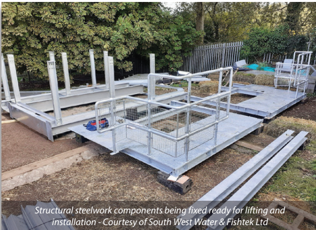
Crane setup within restricted location & approach track Courtesy of South West Water & Fishtek Ltd
