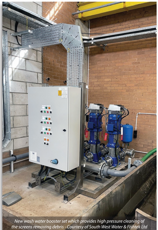
Complete Installation of the S1800 Hydrolox screens and decking system Courtesy of South West Water & Fishtek Ltd
