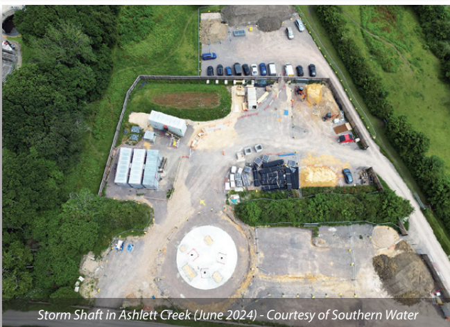
Refurbishment of redundant storm tanks at Millbrook to provide 3,400m 3 capacity - Courtesy of Southern Water
