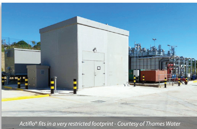
Close up view of the completed Actiflo® AS3 units - Courtesy of Thames Water
