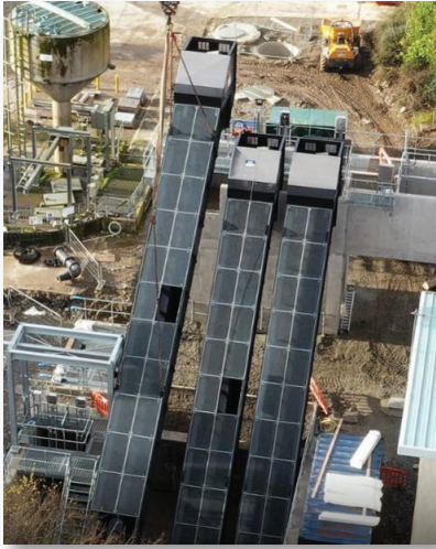
STRABANE WwTW 3 (No.) compact screw pumps supplied, installed and commissioned
