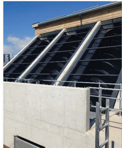
NEW MONKS FARM DRAINAGE PS 3 (No.) screw pumps supplied, installed and commissioned
