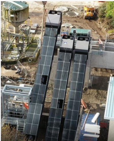
STRABANE WwTW 3 (No.) compact screw pumps supplied, installed and commissioned
