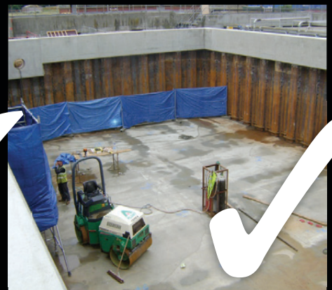
STORM WATER TANKS
