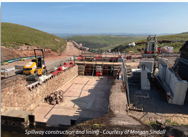
Installation of GRP lining from iLine Technologies Ltd Courtesy of Morgan Sindall
