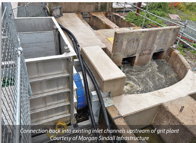
Overpumping manifold to isolate existing inlet works and grit plant Courtesy of Morgan Sindall Infrastructure
