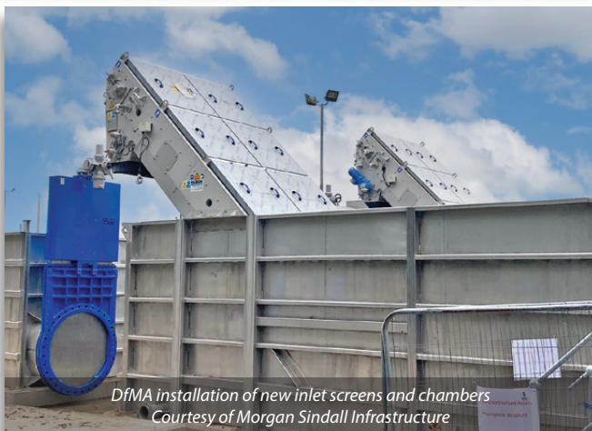
Connection back into existing inlet channels upstream of grit plant Courtesy of Morgan Sindall Infrastructure
