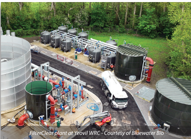
Skid design at Yeovil Pen Mill WRC for easy access and maintenance Courtesy of Bluewater Bio
