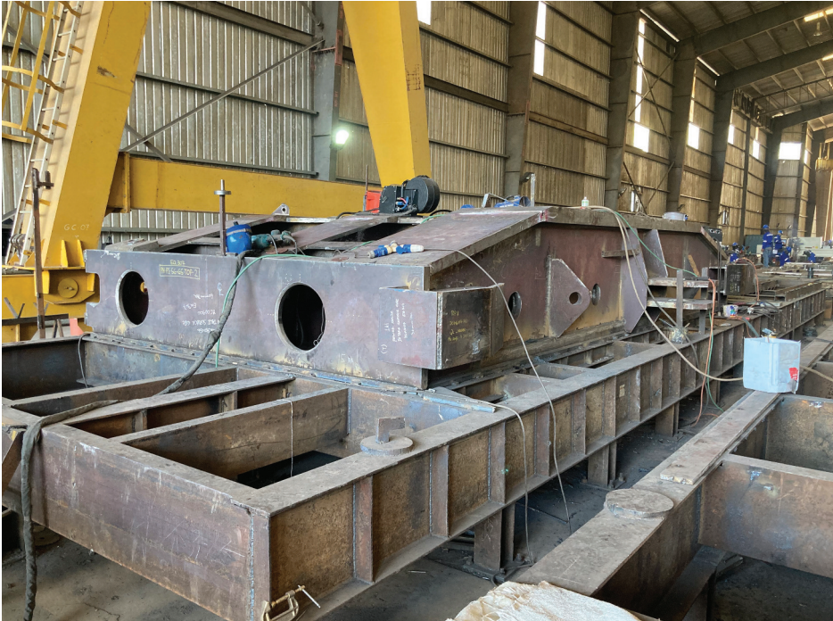
First power intake gate, top section
