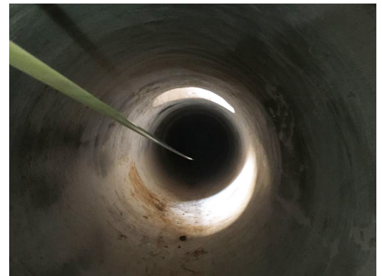
Figure 1. SoundPrint® AFO consisting of a fibre optic cable installed inside the length of the pipeline.
